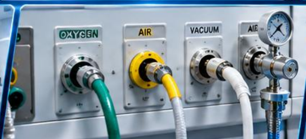
MEDICAL GAS SYSTEMS
